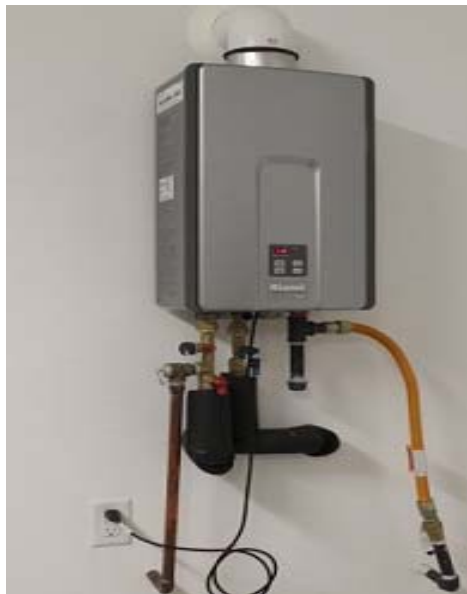
State Housing Law Program Staff Photo: Tankless Water Heater in New Single-Family Home
