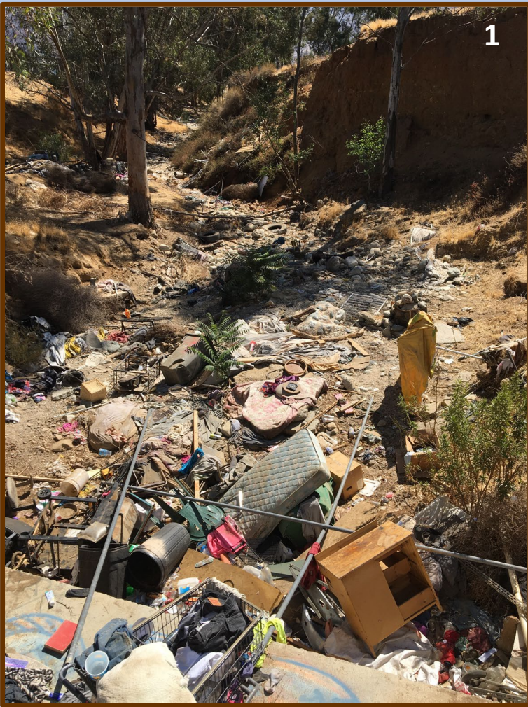
Photo 1 - Creek bed is filled with debris and trash.
